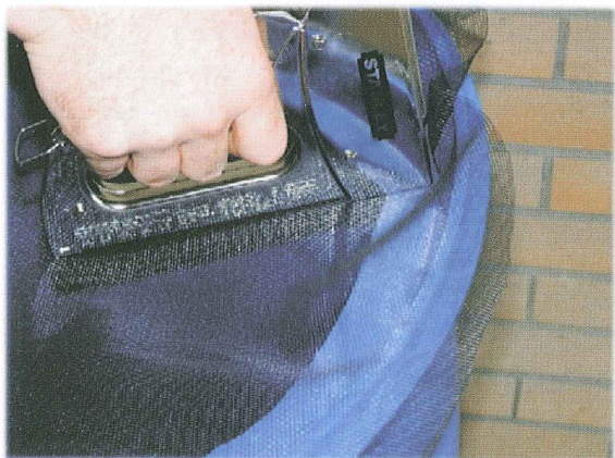
Figure 5. Attach fiberglass screen to the rim on the top of the barrel using a staple gun.
